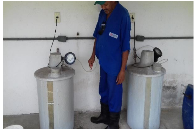
Figure 14: Pumping of caustic soda and chlorine
