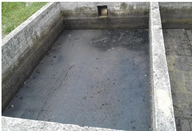
Figure12: Drying sludge bed
