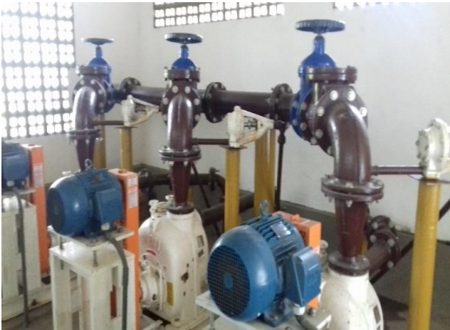
Figure10: Pumping of sewage
