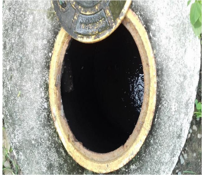
Figure 8: Entrance of sewage in the STS
