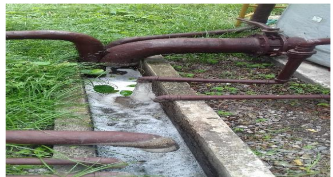
Figure15: Out of treated sewage
