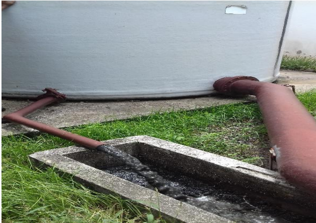
Figure 11: Discharge of sludge in the tank of decantation
